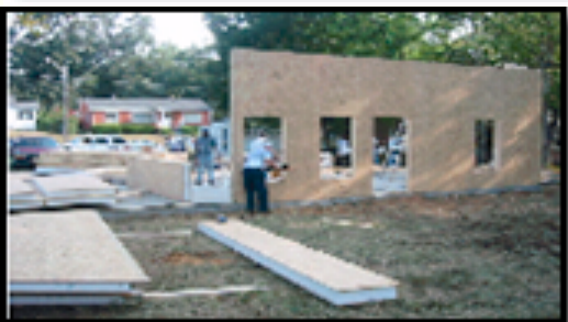
After twenty to forty minutes of work, the exterior walls were more than a quarter complete. All exterior walls were installed in less than three hours.
